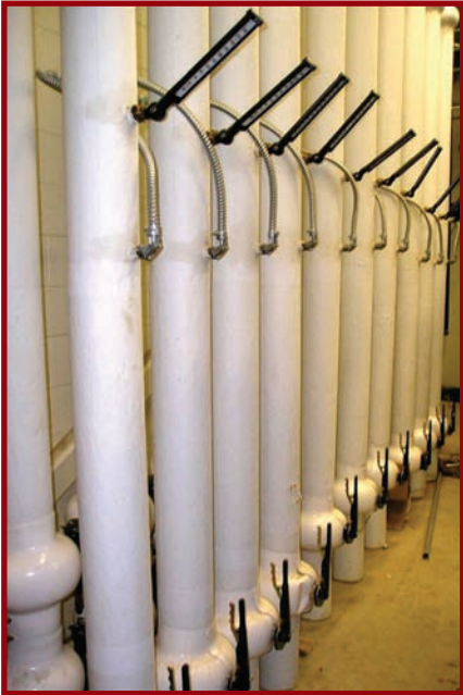
Geexchange supply and return branch mains lined up in the main mechanical room.
