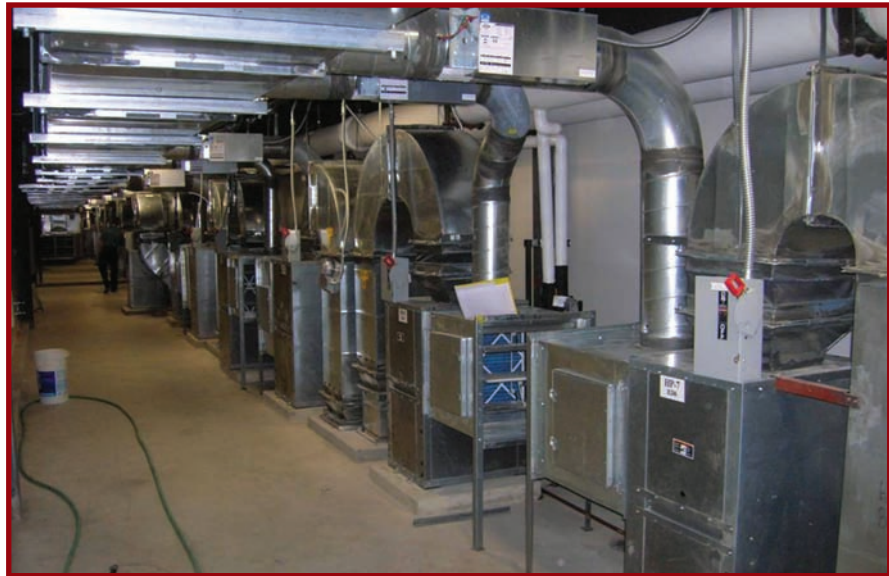
Mechanical mezzanine showing individual heat pumps with air terminal units providing measured quantity of ventilation air.
